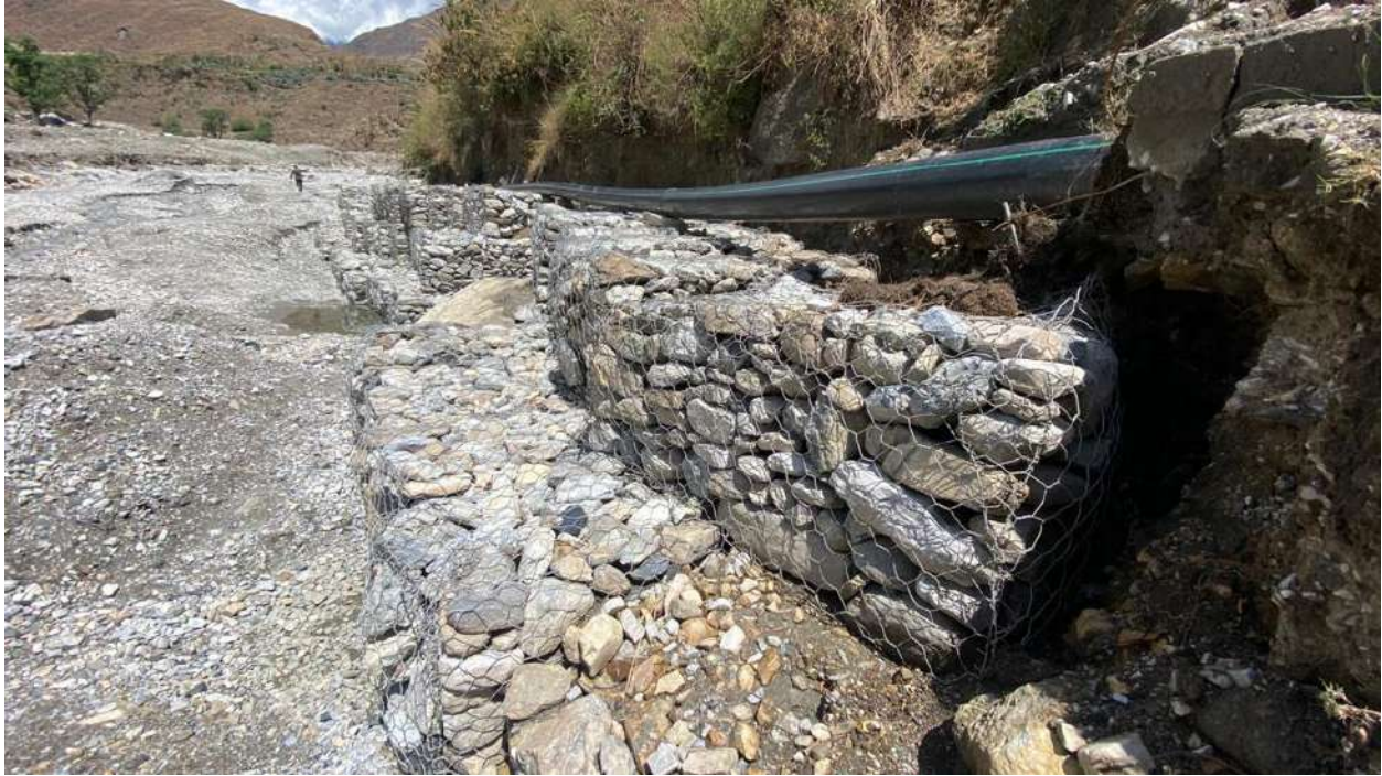
Figure 2: Gabion wall constructed in the starting of Dansaghu Khola, which affects the villages of downstream, Bajedi village is one of them.
